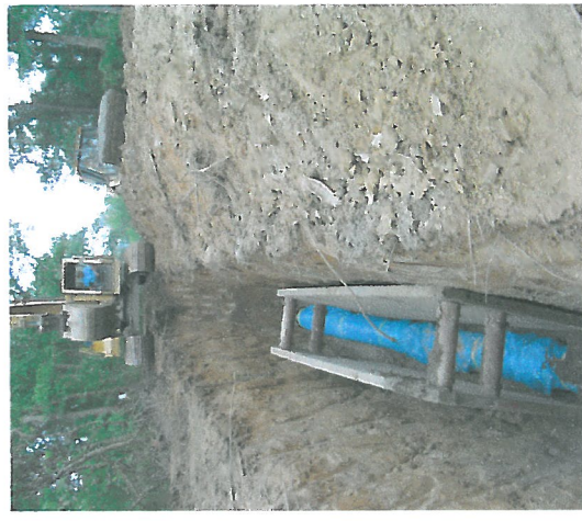
16" Water Main - Bullitt Co., KY
